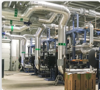
District heating plant facility Sweden, 30 MW
